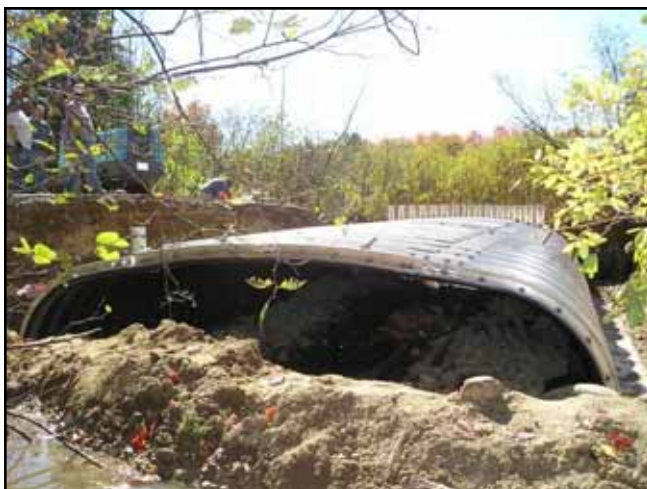
An open bottom culvert is installed in Gray where Totten Road crosses Thayer Brook.
